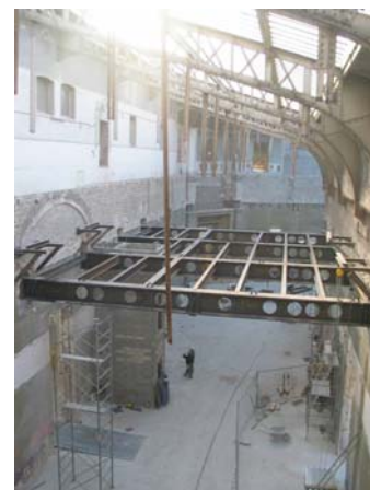
The rehabilitation of the Petit Palais in Paris is an example of reinstatement: strengthening, but retaining the character and the volumes.
