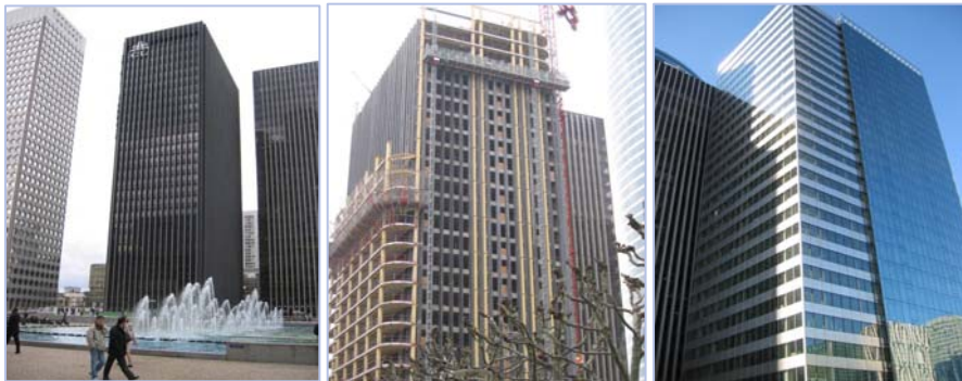
PB12 Tower before (left), during (centre) and after (right) its rehabilitation. The difficulty lay in the height of the building, the very tight timeframe, the need to provide stronger and less bulky load-bearing structures than the original concrete columns: a superlative market for steel.
